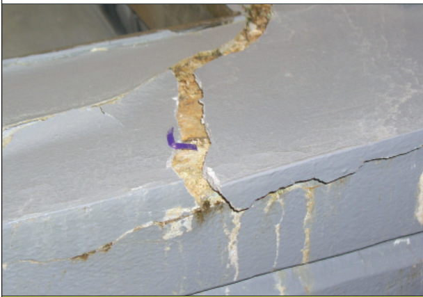
Figure 2. Coating failures and pH irregularity caused cracks in this floor.
